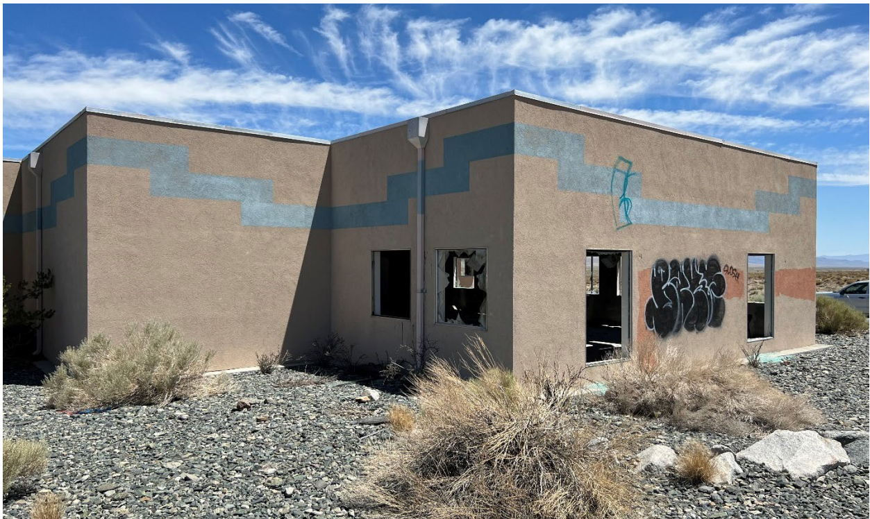
Figure 12. Northwest corner of the building showing additional broken windows.
