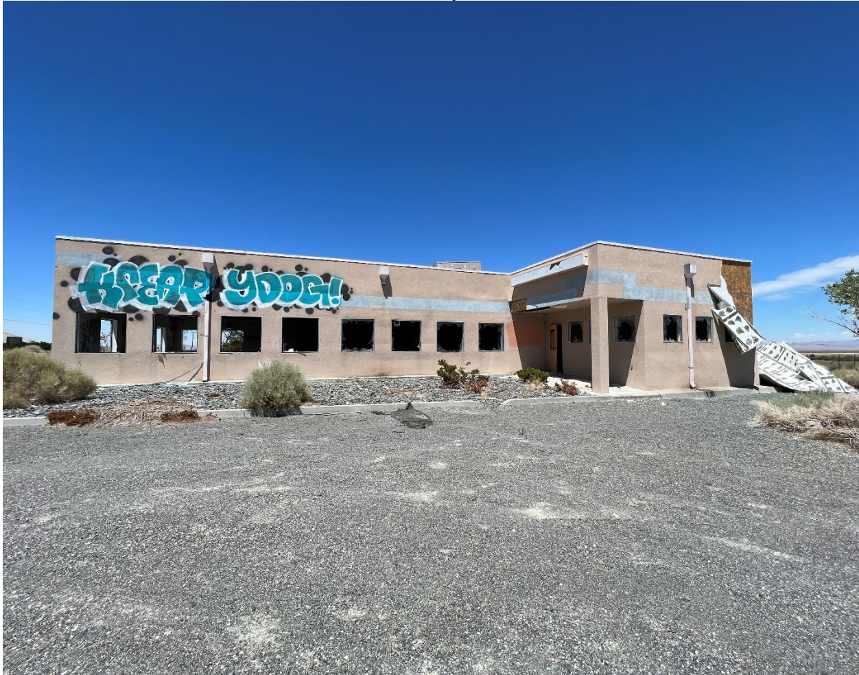
Figure 1. Abandoned truck stop located on the Walker River Reservation and south of Schurz.
