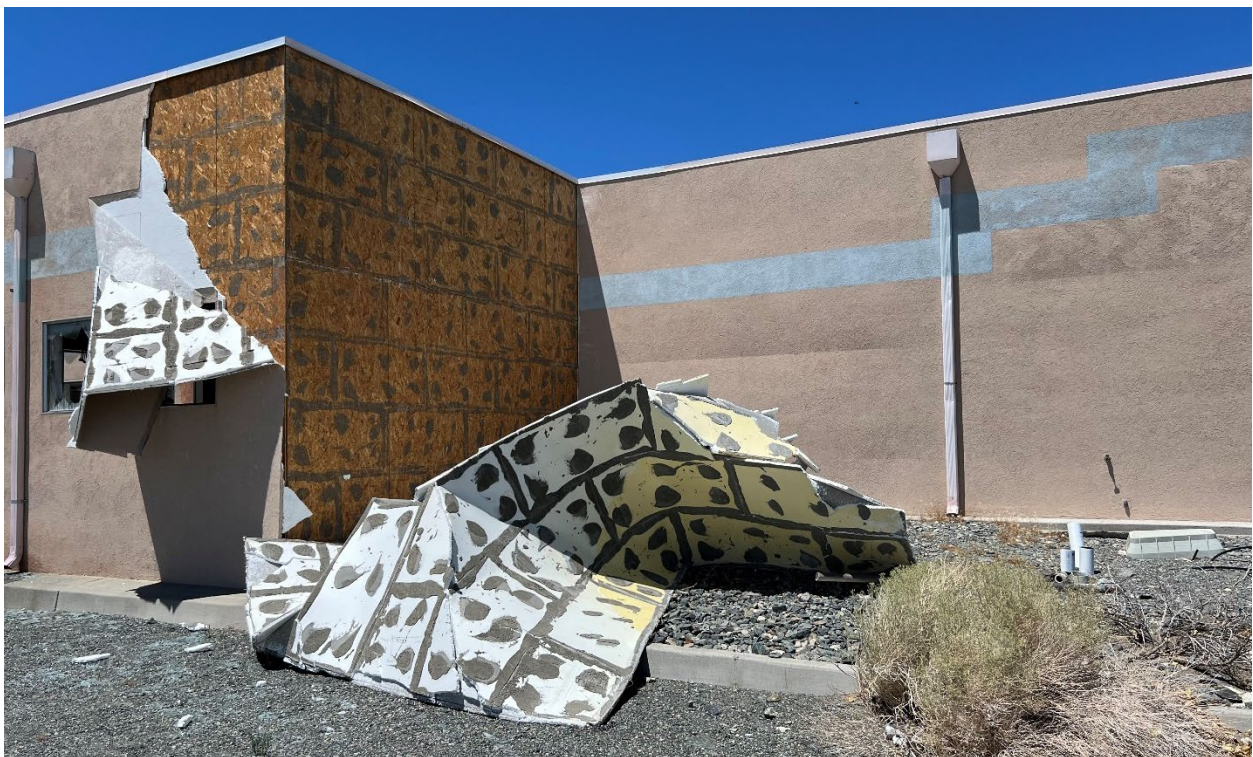
Figure 8. Southeast corner of the building with detached siding material.
