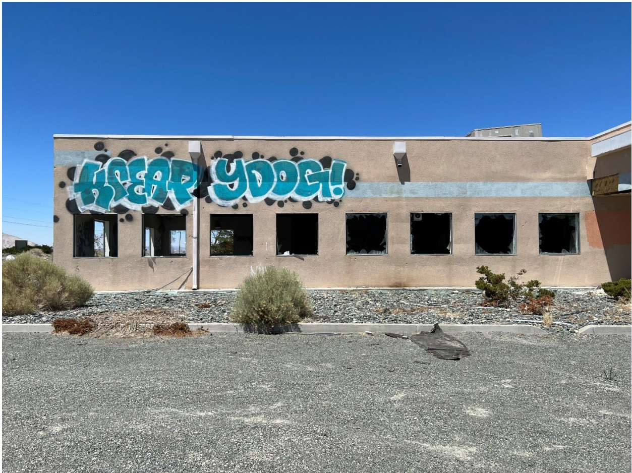
Figure 4. South exterior side of the old truck stop showing broken windows and vandalism.
