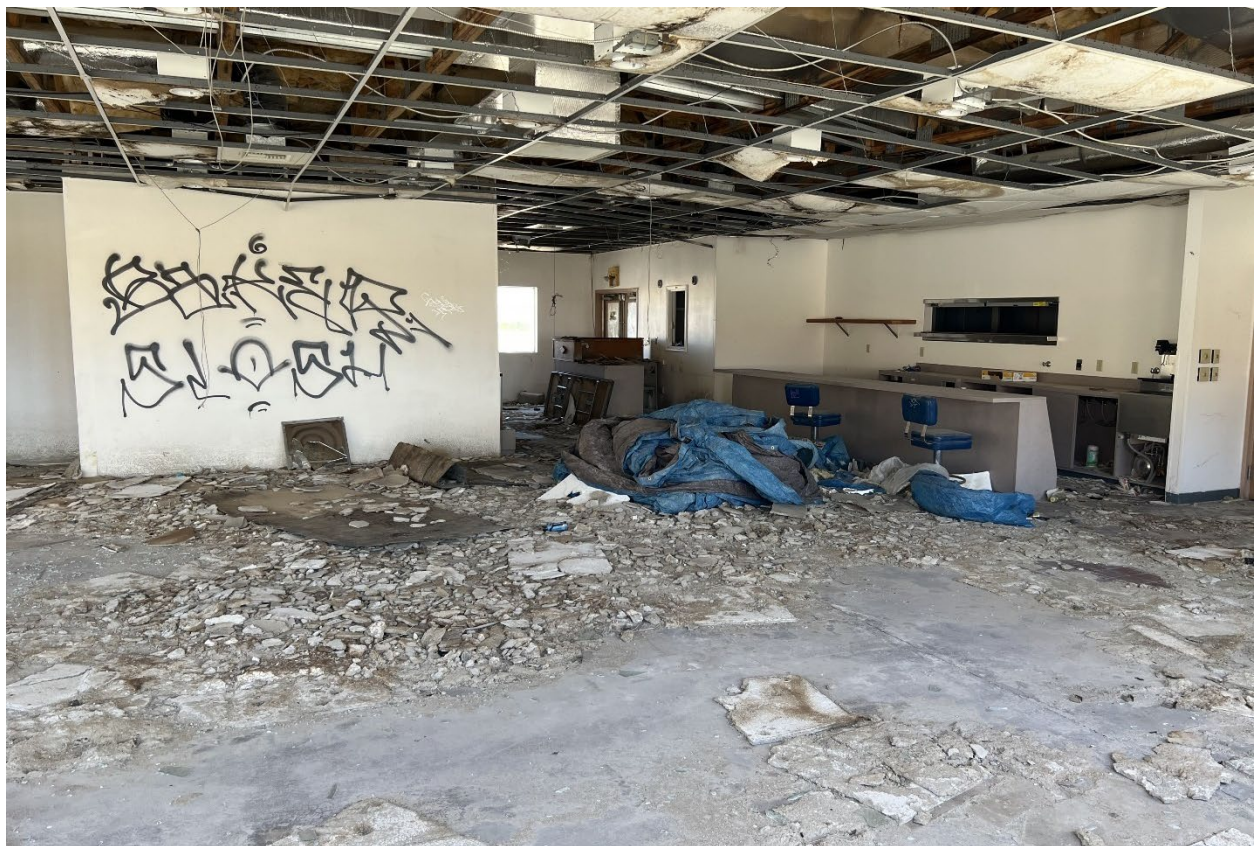
Figure 6. Common area interior space of the structure showing the bar and rear kitchen area.
